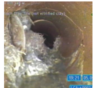
Structural failure observed on Oak Street
