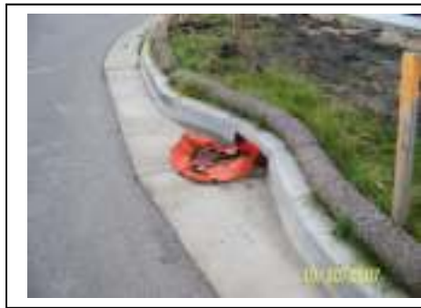
Street Inlet Protection
