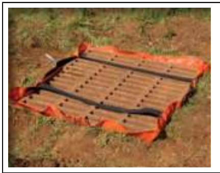
Drop down inlet protection device
