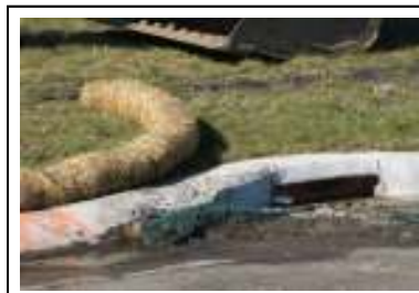
Damaged inlet protection
