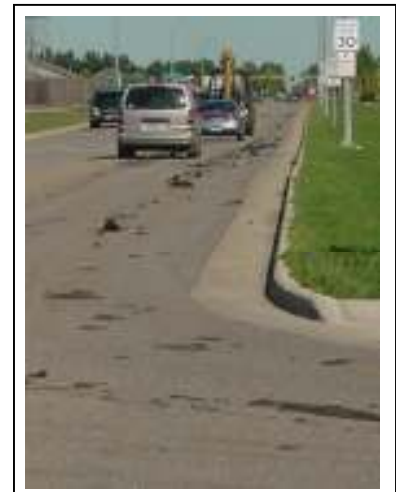
Sediment tracked onto roadway
