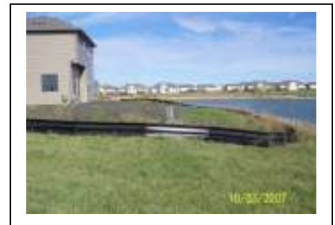
Silt fence on a residential site
